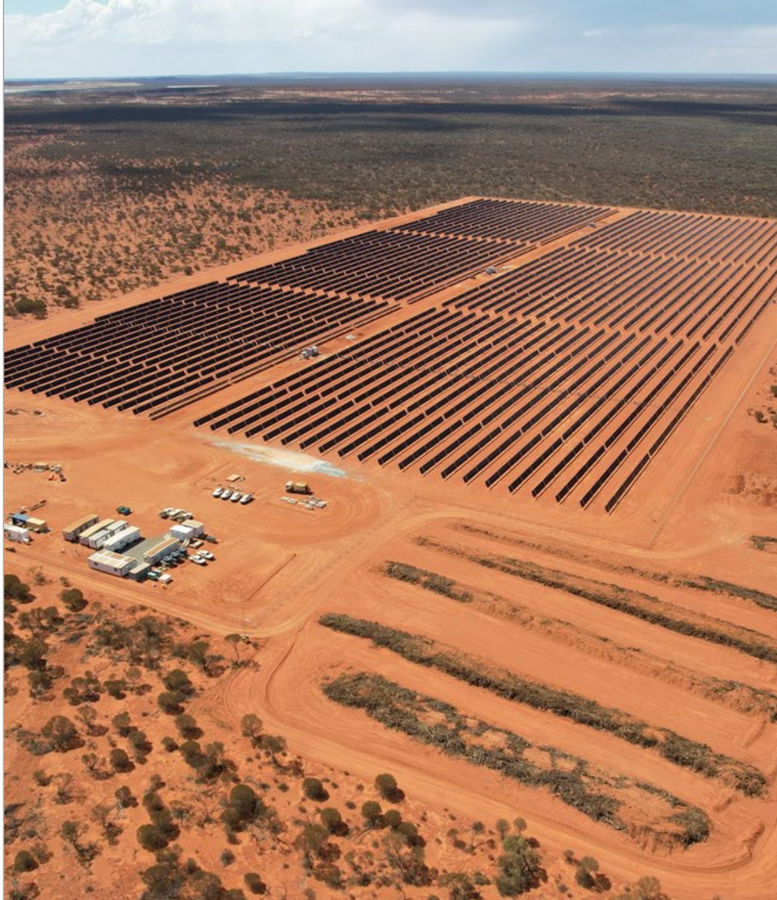
Northern Goldfields Solar Project Leinster, Australia
